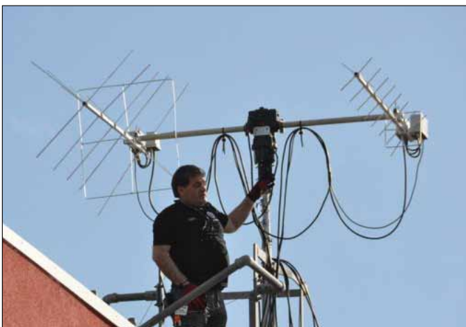
► Ciaran, M0XTD checks the connections on the VHF and UHF beams on the roof of the school
