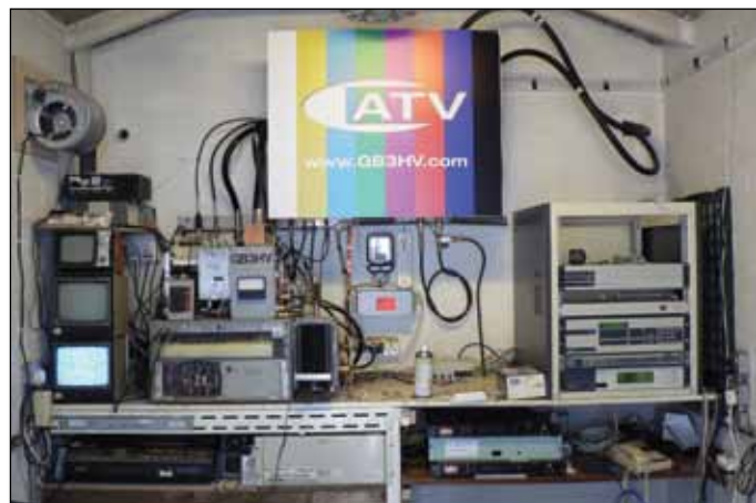
▶ Digital equipment installed at GB3HV
