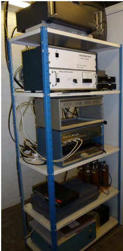
Fig.9. Equipment Rack at GB3TM
