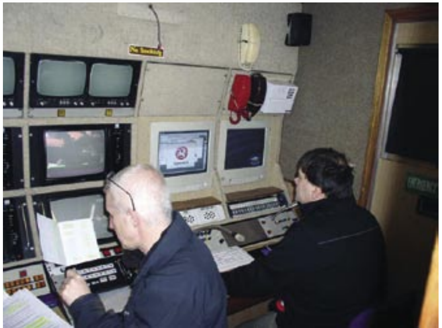
The control room
