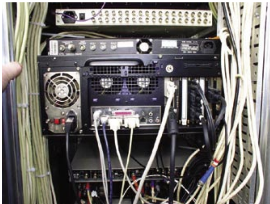
A rear view of the VT computer
