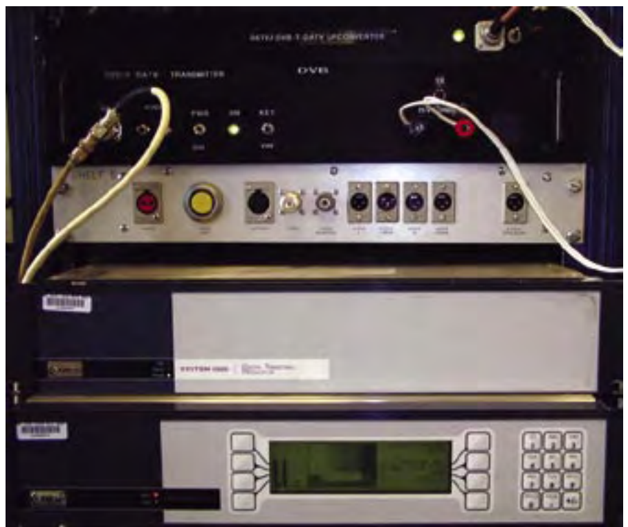
DVB-T Transmit Equipment
