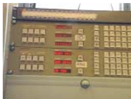
Control panel, Matrix
