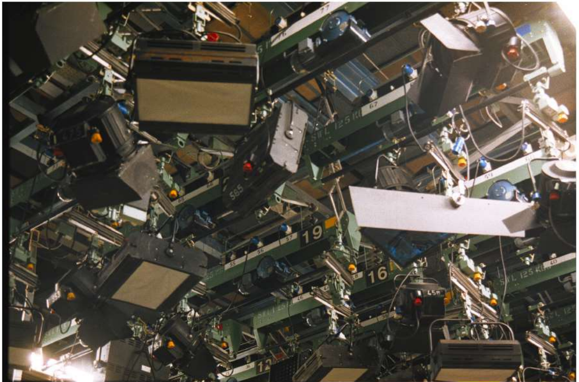
The Maidstone Studios, lighting boat system supports 6-10 lanterns. The lighting boat is supported by steel cables wound onto 2 motorised drums.
