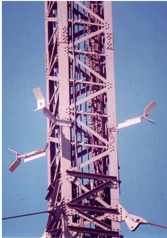
The three through-reflector antenna used by Dartmoor repeater GB3WV
